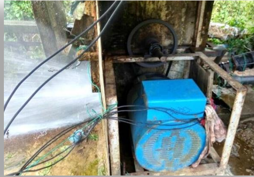
Micro Hydro System for Puneng Trusan village in Sarawak
